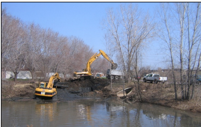
Ponds are designed to detain or retain stormwater and slow the rate of outflow
