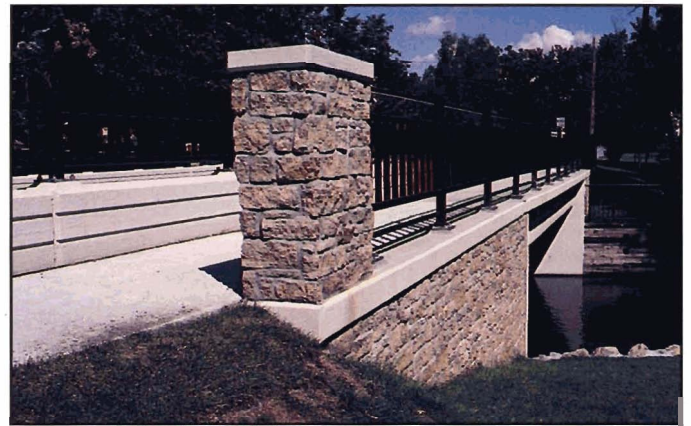
Fig. 6-8. Combination of parapet and light metal pedestrian railing address both functional requirements and appearance, Minneapolis, Minnesota
