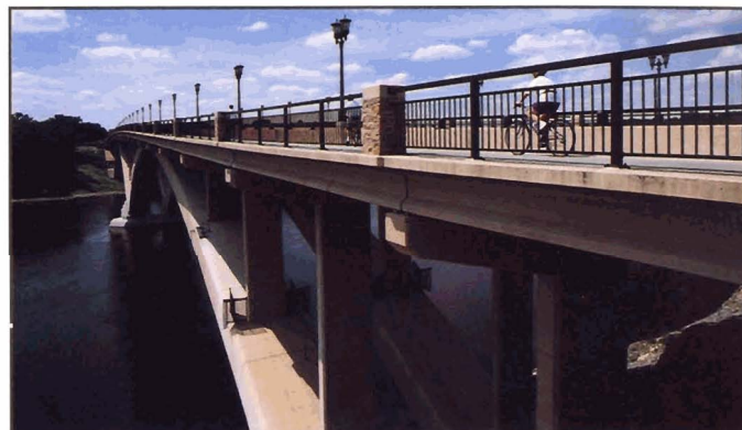
Fig. 6-4. Parapet and pedestrian railing designed to allow drivers to see through, allowing a view of the scenic area, Lake St. Bridge, St. Paul/Minneapolis, Minnesota
