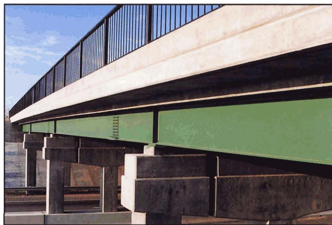
Fig. 7-10. Bridge widening – newly constructed piers adjacent to initial construction emulate the visual design of the initial design
