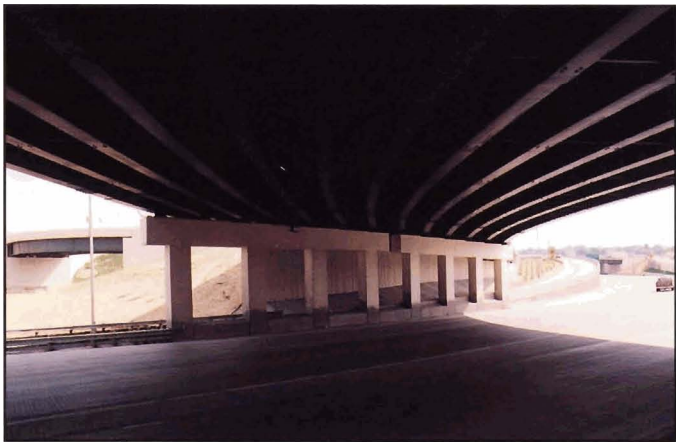
Fig. 6-12. Bottom flange lines dominate view of bridge from below, providing a clean appearance
