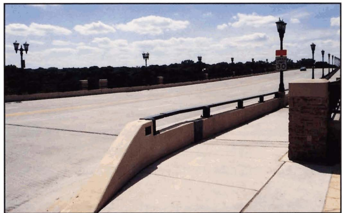
Fig. 6-6. Barrier transition provides logical and smooth progression from curb to parapet, Lake St./Marshall Ave. Bridge, St. Paul/Minneapolis, Minnesota
