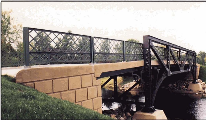
Fig. 6-21. Buff-colored concrete in combination with separate finish colors for railing and structure provides visual interest, Island Canal Bridge, St. Paul, Minnesota
