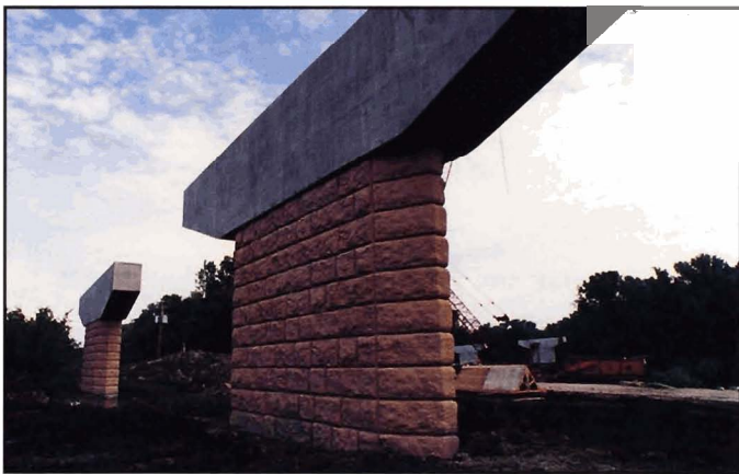
Fig. 6-26. Simulated cut stone pattern and coloring on pier shaft, Bloomington Ferry Bridge, Bloomington, Minnesota
