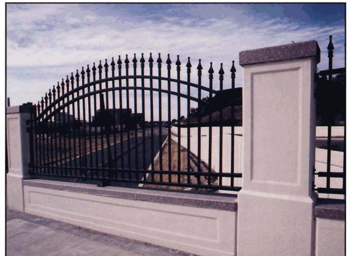
Fig. 6-9. Use of stone caps, concrete balusters, recessed panels, and picket railing adds to architectural flavor of bridge, St. Paul, Minnesota
