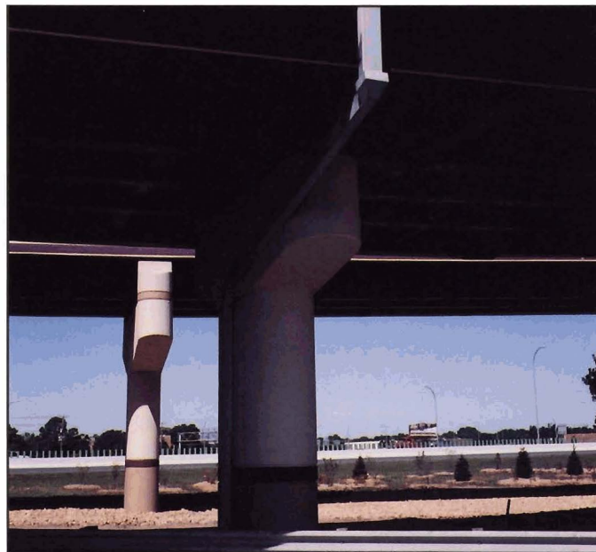
Fig. 6-13. Drain pipe placed on opposite side of pier from oncoming traffic and follows fundamental shape of pier
