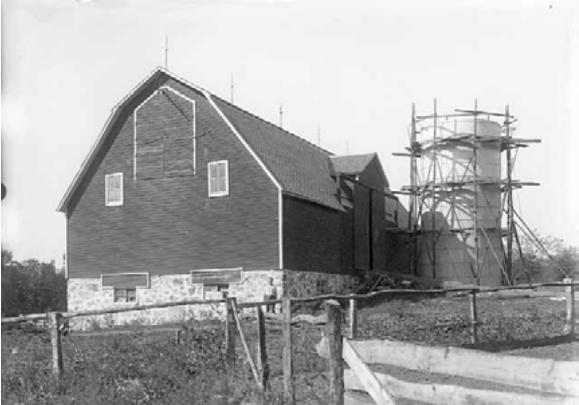
Silo under construction next to barn. Location unknown, circa 1920. (MHS Neg. No. 11077-A)
