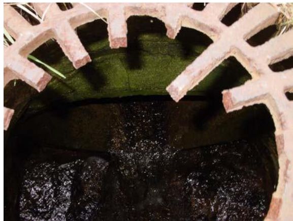
FIGURE 12: SEVERE GRATE DAMAGE
