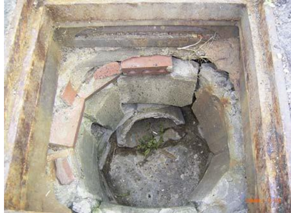
FIGURE 10: DAMAGED MANHOLE IN NEED OF REPAIR
