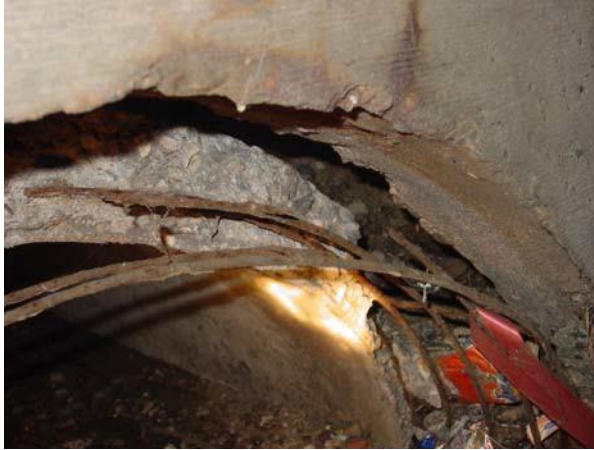
FIGURE 6: PCC CULVERT JOINT FAILURE
