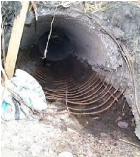
FIGURE 8: SEVERE PCC CULVERT DAMAGE
