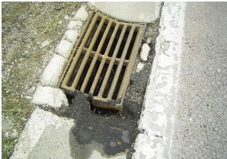
FIGURE 14: CURB DAMAGE AT INLET GRATE
