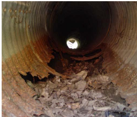
FIGURE 7: CORRUGATED METAL PIPE (CMP) RUSTED AND BENT IN NEED OF REPAIR OR REPLACEMENT
