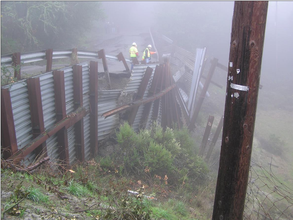
Figure 2-17: Sonoma Mountain Road Retaining Wall Failure in 2008
