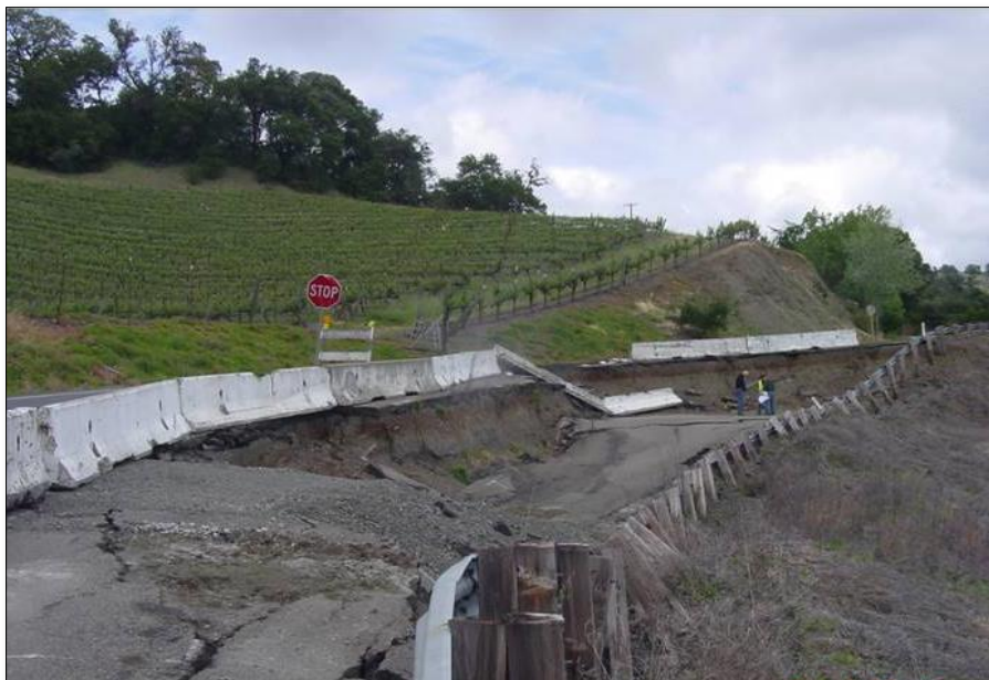
Figure 2-21: Landslide at Geysers Road, Sonoma County
