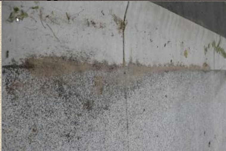
Fairly Clogged Location
