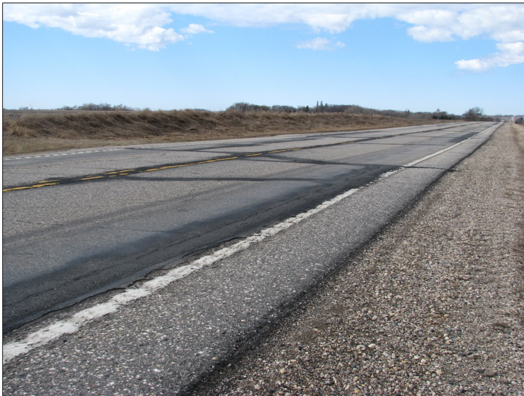
Figure 9: Poor Pavement Quality Caused by Ice Heaves
