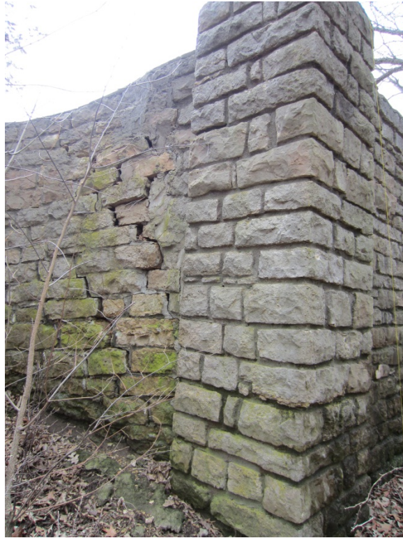
4.6 – Cracks indicating movement of the wall
