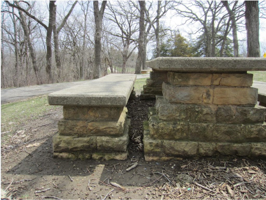
4.8 – Dirt and moss on West Table
