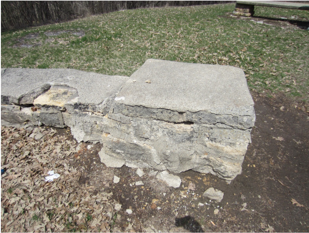
4.7 – Significant deterioration at wall and pier of East Overlook Wall
