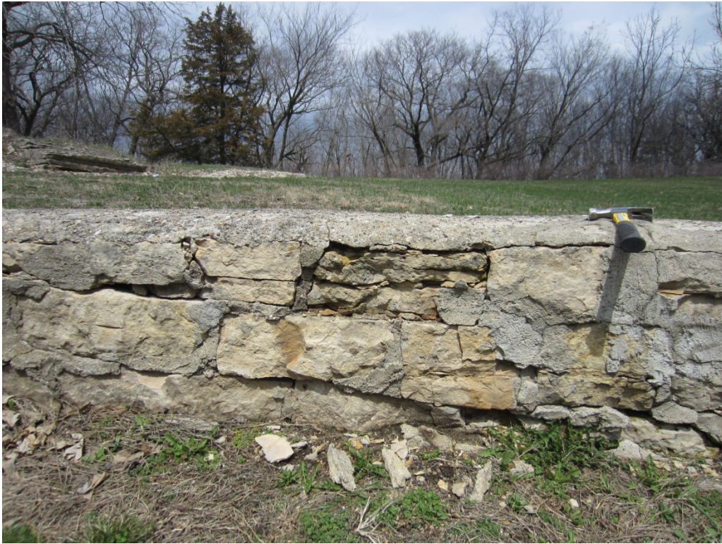
4.5 – Dry laid freestanding masonry of South Entrance walls showing mortar cap, mortared joints, and stone deterioration
