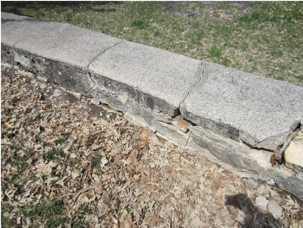
4.7 – Mortared cap, joints, and stone deterioration at East Overlook Wall
