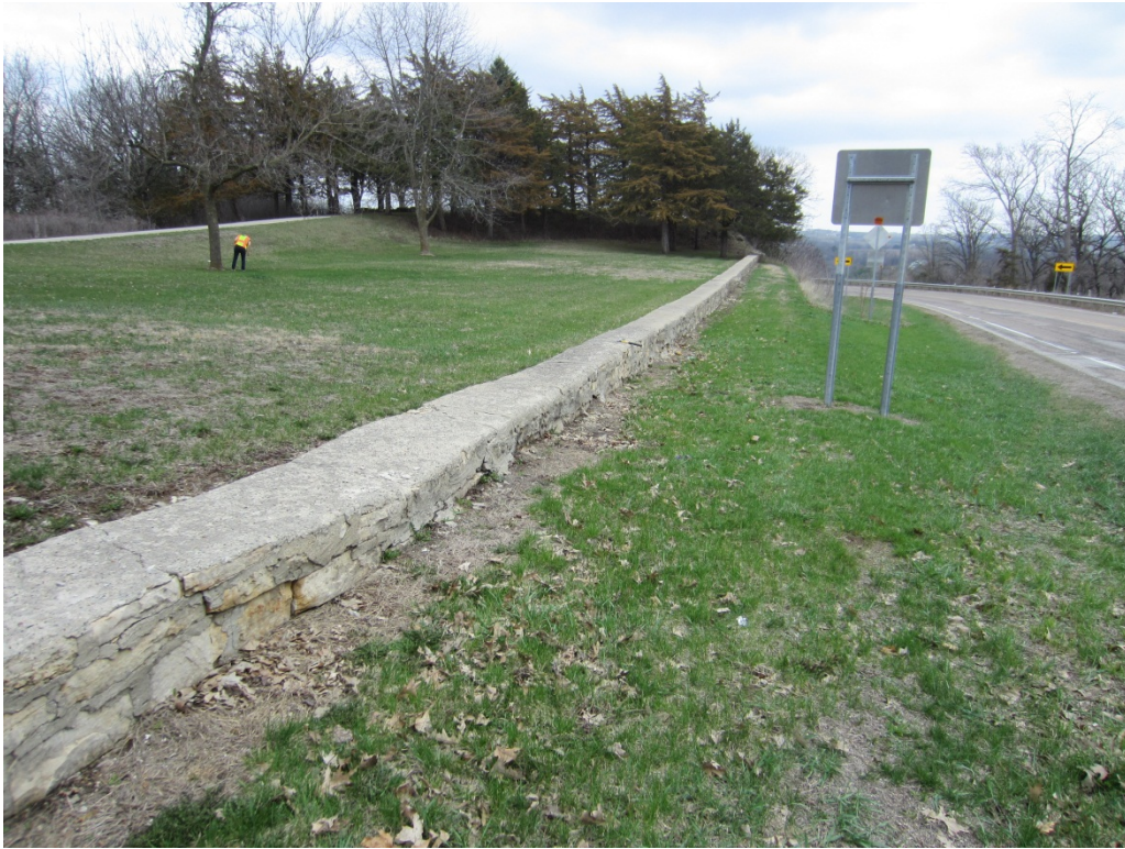
4.5 – Shifted sections of East Entrance Walls
