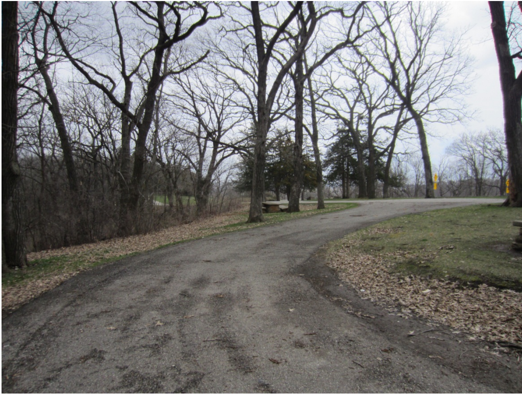
4.2 – West Drive with deteriorated and cracking bituminous
