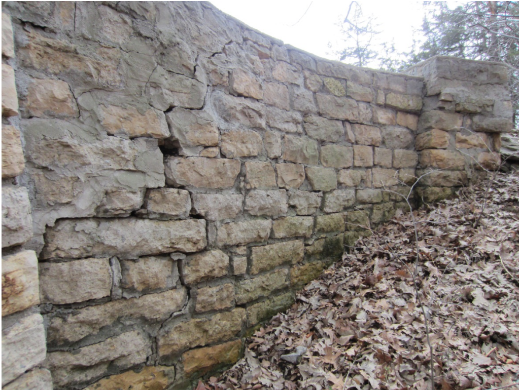
4.6 – Cracks indicating movement of the wall
