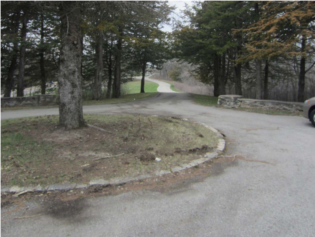
4.7 – Flush curbstones and tree at the island of the East Overlook Wall and Parking Area
