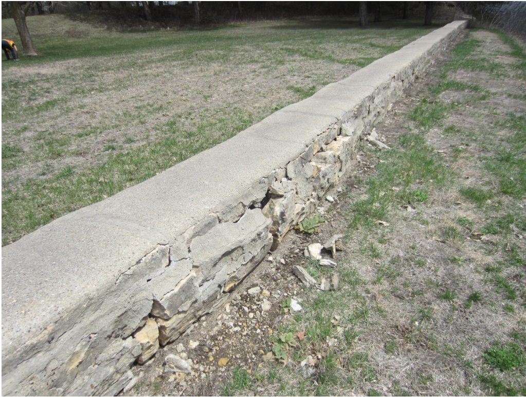
4.5 – Significant deterioration at South Entrance Walls
