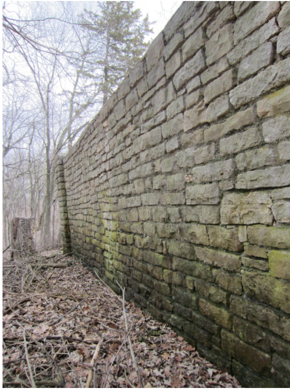
4.6 – North Overlook Retaining Wall – note tilting of the wall from plumb
